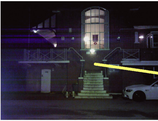
Bldng. heat Loss via wall damage / crack !
