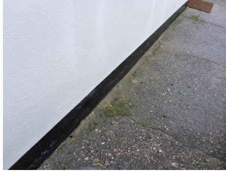
Render is in direct contact with the ground
