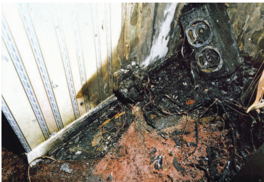
A typical fire of electrical origin caused by a number of plugs connecting an audio system and several other appliances drawing excessive current and overloading a single socket.
