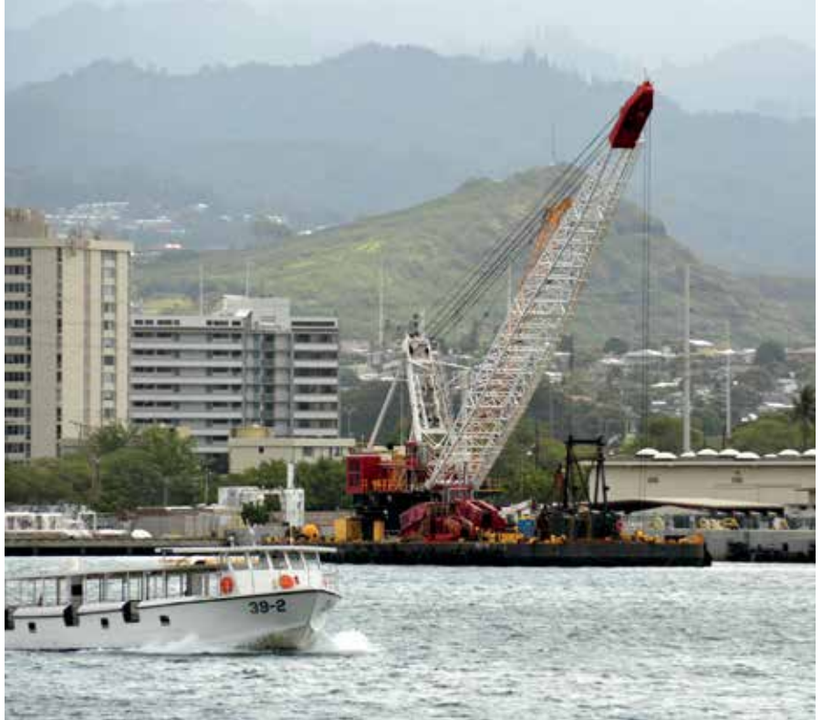
Watts-Healy Tibbitts A JV dredging the harbor alongside JBPHH's piers. PHOTO COURTESY DENISE EMSLEY/NAVFAC HAWAII PUBLIC AFFAIRS
