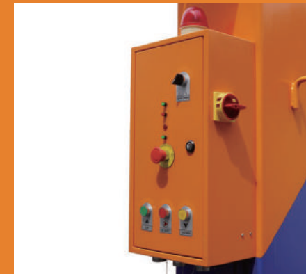
Each column is equipped with an emergency stop button.
