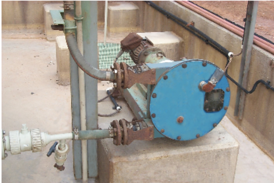
Hydrochloric Acid Pump
