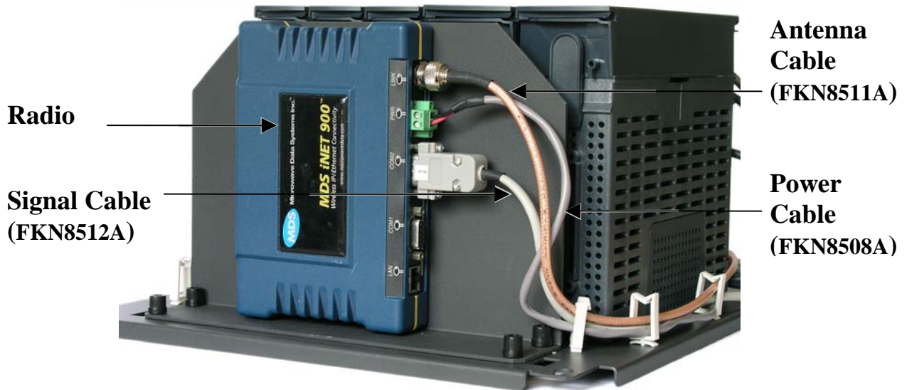
Figure 13-48 iNET 900 Radio Modem Installed on ACE3600 Chassis – Cable Connections
