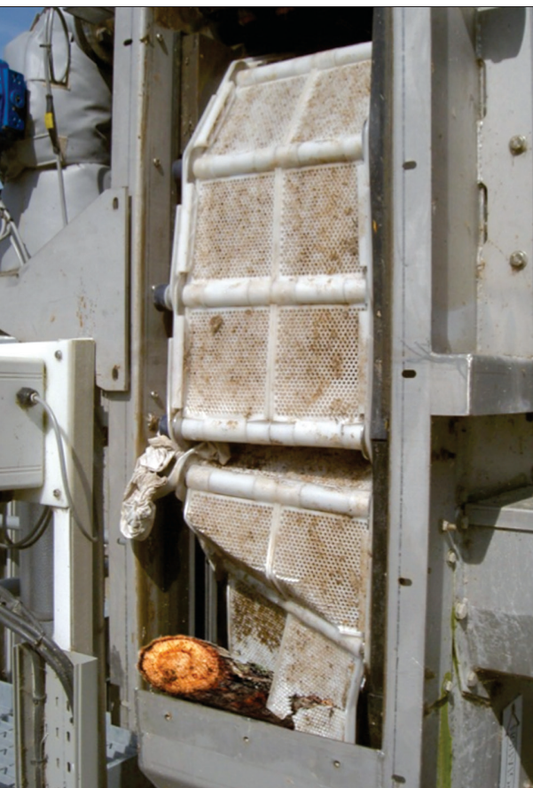
Damaged inlet screen
