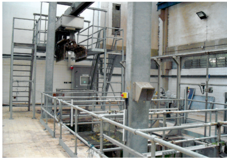
Bosker Overhead Trashrake at Thames Water's Deephams wwtp.
