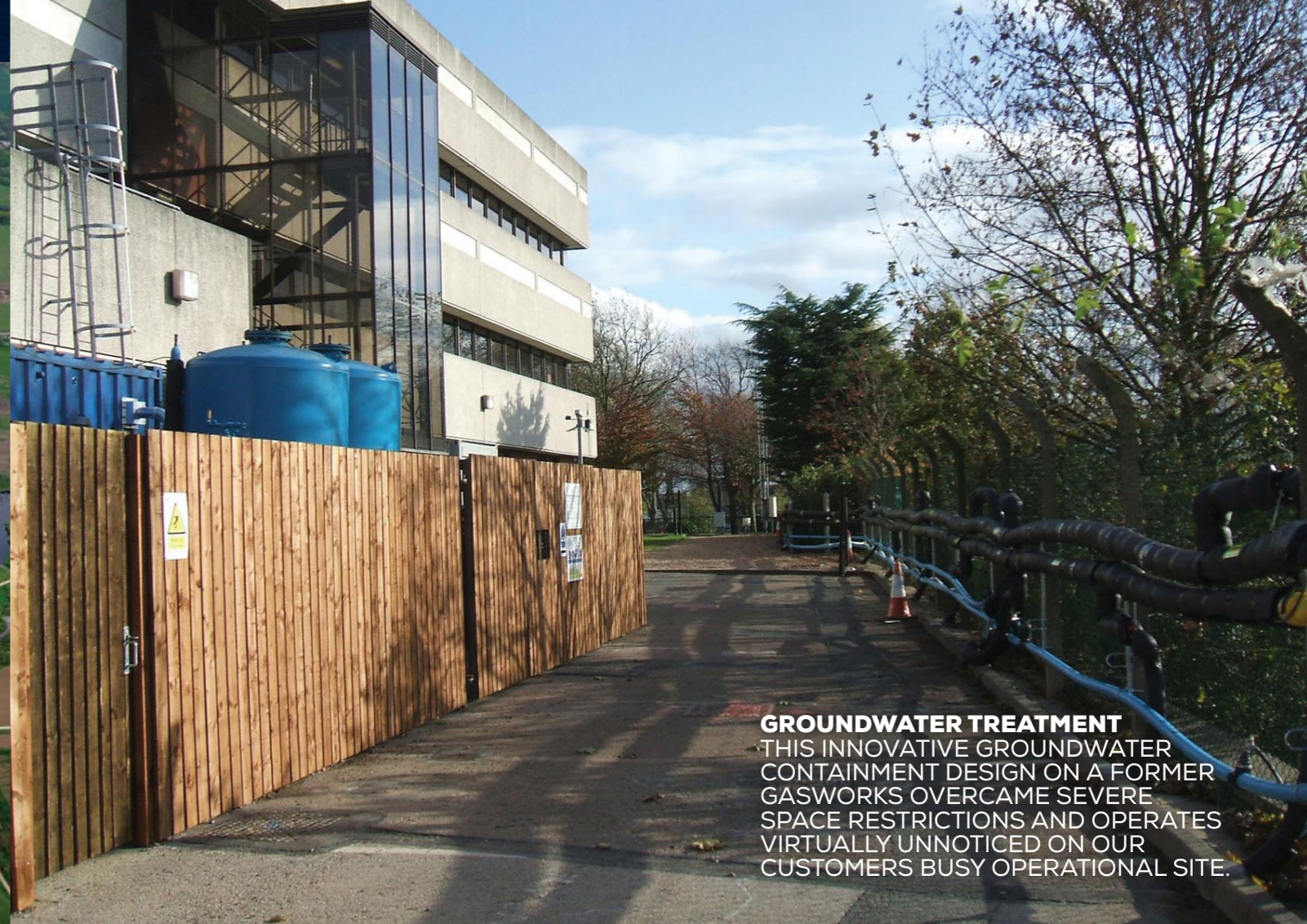
RAYNESWAY RESOURCE PARK, DERBY THE UK'S LARGEST CHLORINATED SOLVENT CHEMICAL OXIDATION PROJECT, DESIGNED AND IMPLEMENTED BY CELTIC AND DELIVERED TO COST AND PROGRAMME AS PART OF A £175M REDEVELOPMENT SCHEME.
