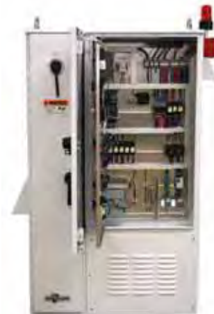
Zone 3: Controls Compartment
