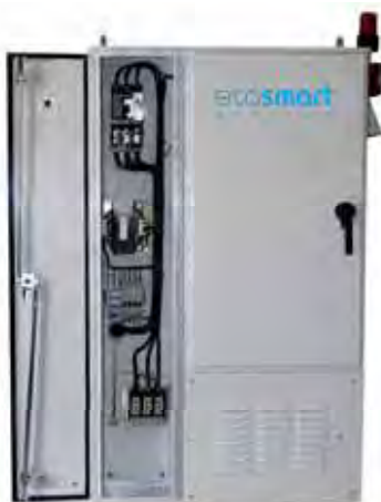
Zone 1: Service Entrance Compartment
