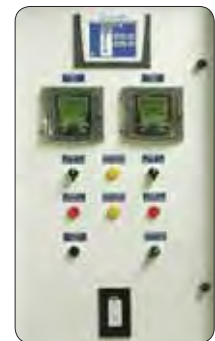
Zone 3: Inner Door of Controls Compartment
