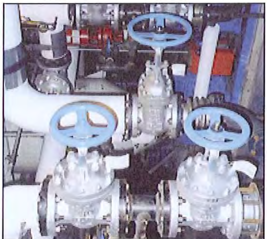
API 600 gate valves in service for a boiler feed installation.
