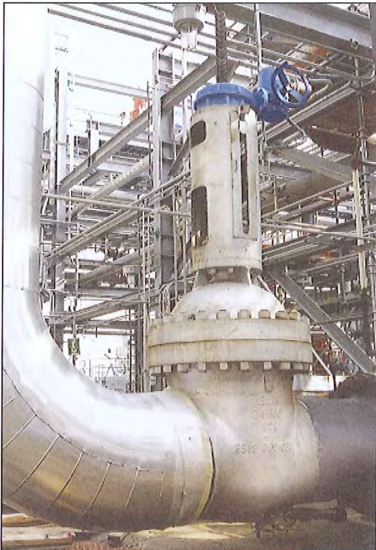
Carbon steel gate valve (ASME Class 600), used for boiler feed water installation at a Hydrogen Plant in Texas.
