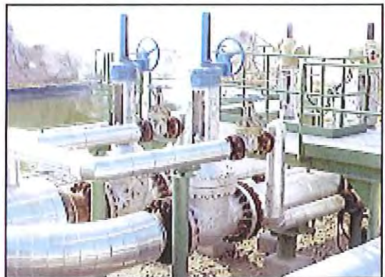
A geothermal power plant valve installation for sour gas service.
