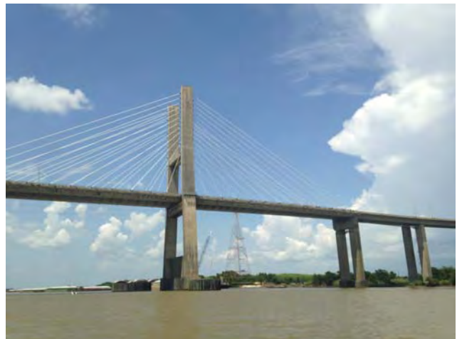
The Cochrane Africatown USA Bridge built in 1990 is a major gateway into the community
