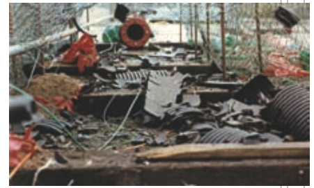
Aftermath of Pipeline from Internal Gas Detonation
