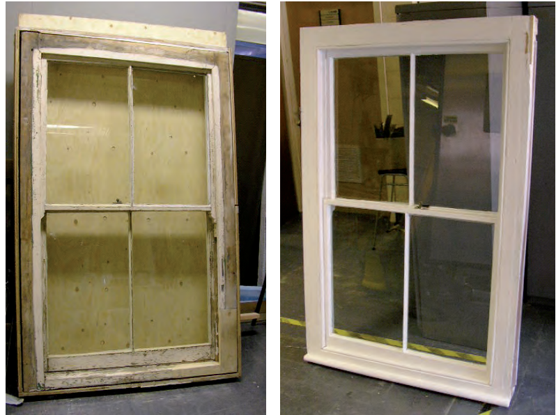
Above left: Window after joinery repairs; right after gap filling and coating with white primer
