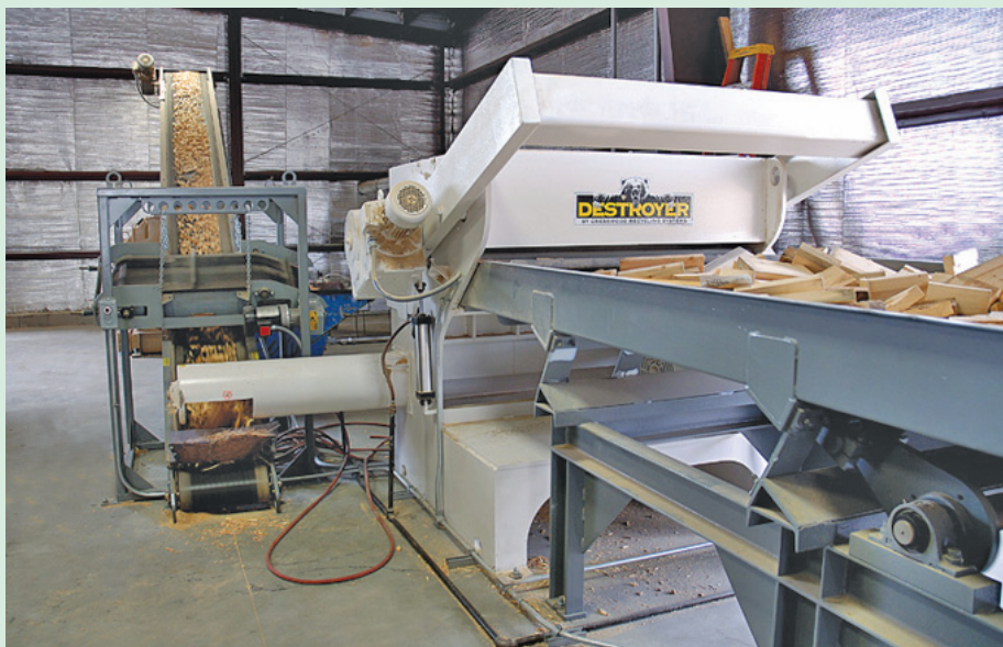
A Cresswood EF-60 “Destroyer” wood grinder processes whole pallets and scrap material into high-value uniform wood chips at the FCA Coal Valley facility.
