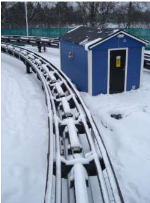
Figure 3. The test track with “double density” linear motors in the acceleration ramp out from the station in Swedish winter weather. The blue building contains the electrical equipment and the propulsion inverters, and cables are routed from the building to each LIM. In a commercial application this will all be integrated into the track using custom- built, small size inverters fully utilizing the short duty cycle for each LIM.
