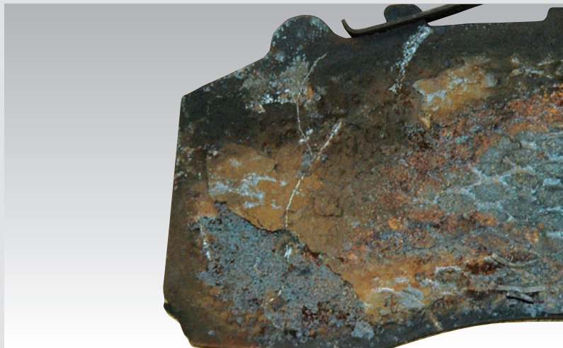
► Heavy underlying corrosion
