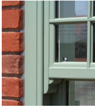
Run through sash horns
