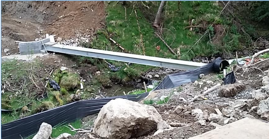
Photo 1: example of an (unfinished) pipe-bridge encased within structural beam. Gangway and handrails would be mounted above and the banks landscaped.
