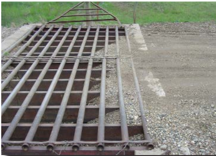
Care must be taken not to spill gravel into the cattle guard. Poor quality gravel with too much loose aggregate aggravates the problem of material spilling into the cavity.
