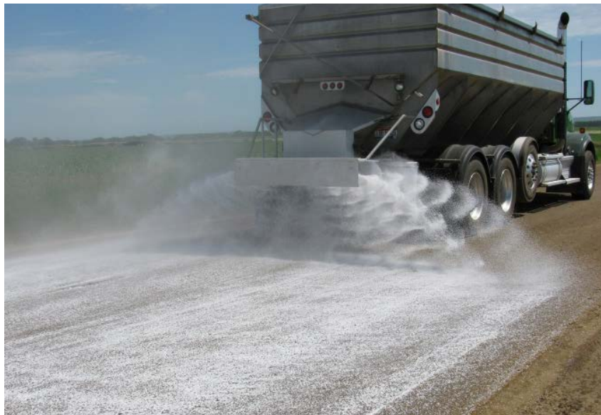
Good example of even application of chloride in dry form – cannot be done in windy conditions.
