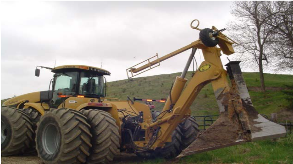
This large tile plow was brought in which is commonly used in some regions to install polyethylene pipe into farm fields for drainage purposes. This type of machine has also been used to plow drain tile into gravel roads with great success.
