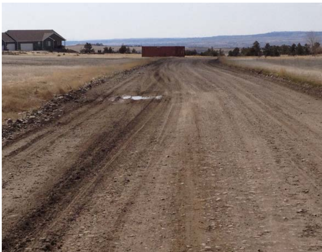
This road has a poor cross section. Drainage is important, even though the road is located in a semi-arid region.
