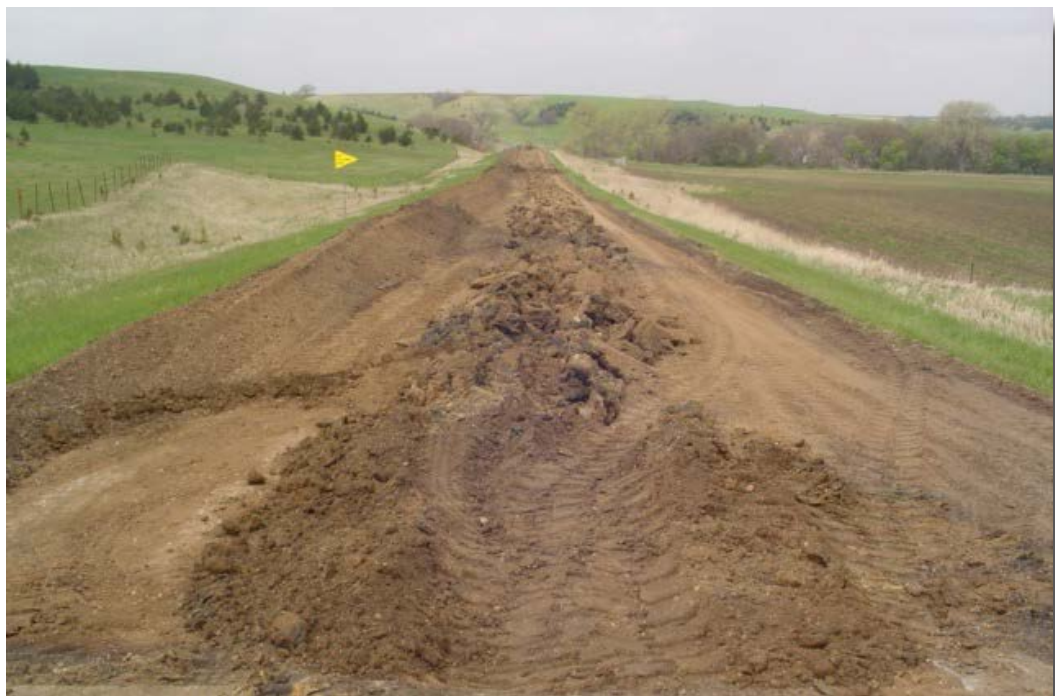
A road that had a constant problem with water percolating upward from springs beneath the surface. Work has just been completed to plow drainage pipe into the subgrade of this road.
