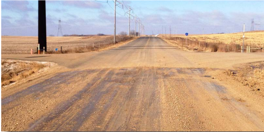
Another area prone to develop washboard or potholes is a transition from gravel to paved surface.
