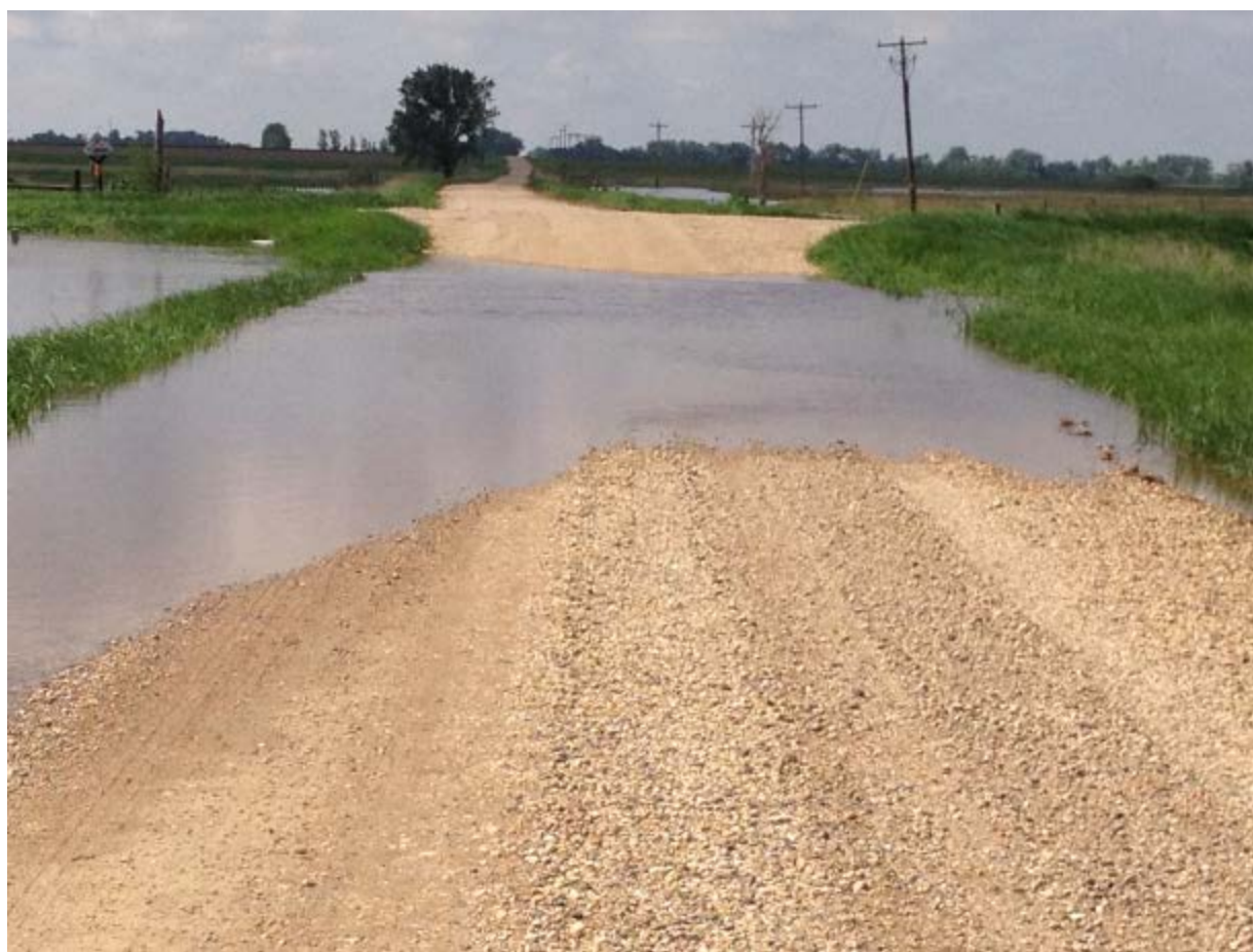
Plugged or collapsed culverts cause serious damage when water flows over roads.
