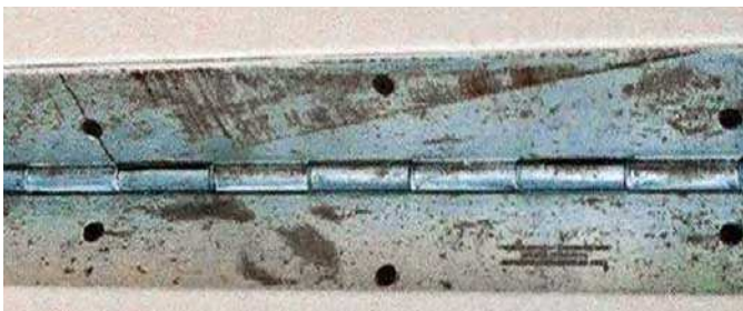
Figure 5: Carbon steel brushes were used by a cleaning contractor on this stainless steel door hinge that was installed beside an indoor swimming pool. The areas with carbon steel contamination are rusting. Photo courtesy of TMR Consulting
