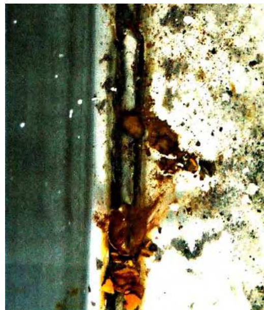
Figure 6: This weld within a swimming pool gutter was not cleaned properly and pitting corrosion is occurring along the weld seam. Photo courtesy of TMR Consulting
