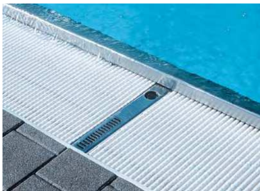
Figure 10 and 11: Type 316 pool gutters and water jet openings in the floor plates. Photos courtesy of Martina Helzel
