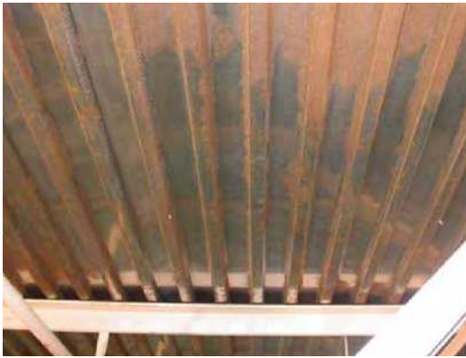
Figure 12: Corrosion of a Type 304 stainless steel roof deck above an indoor swimming pool. Photo courtesy TMR Consulting
