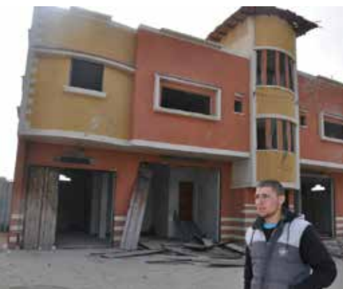
Destruction Remnants of a House belonging to al-Najjar Family after Israeli Airstrike on the area
