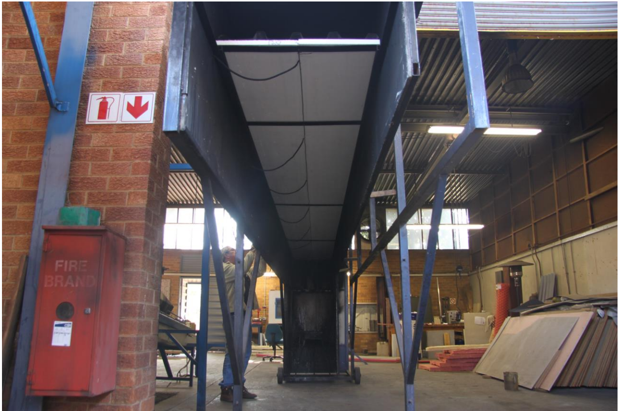
Figure 4.2.1.1: The test installation prior to ignition of the Fire Source
