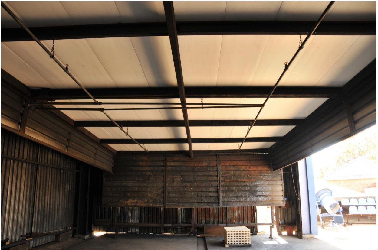
Figure 4.3.1: The SANS 10177-11 test installation prior to ignition of the Fire Source
