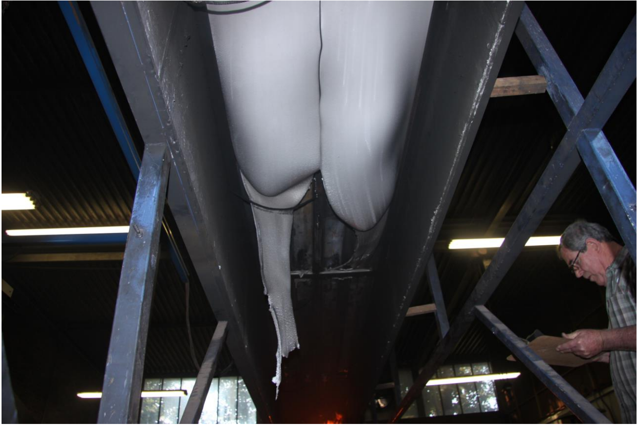
Figure 4.2.3.7: Heat damage up to 6 meter mark with material dropping out
