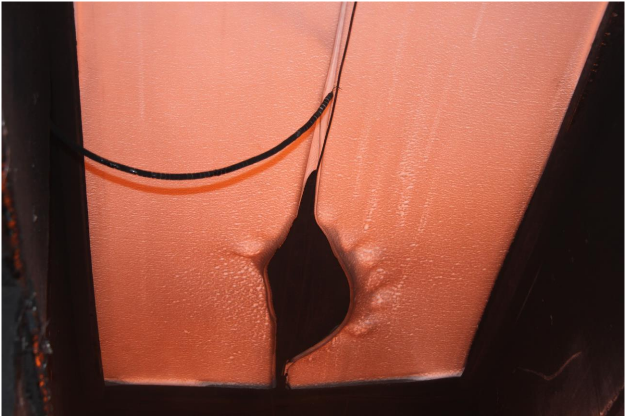
Figure 4.2.3.3: Material discolouring with joint opening above Fire Source
