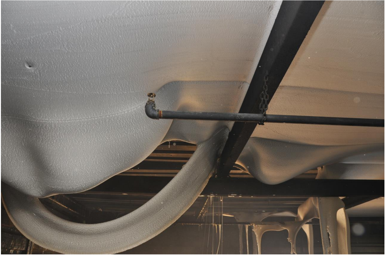
Figure 4.3.9: Material draping close to sprinkler head and over sprinkler pipes in rear
