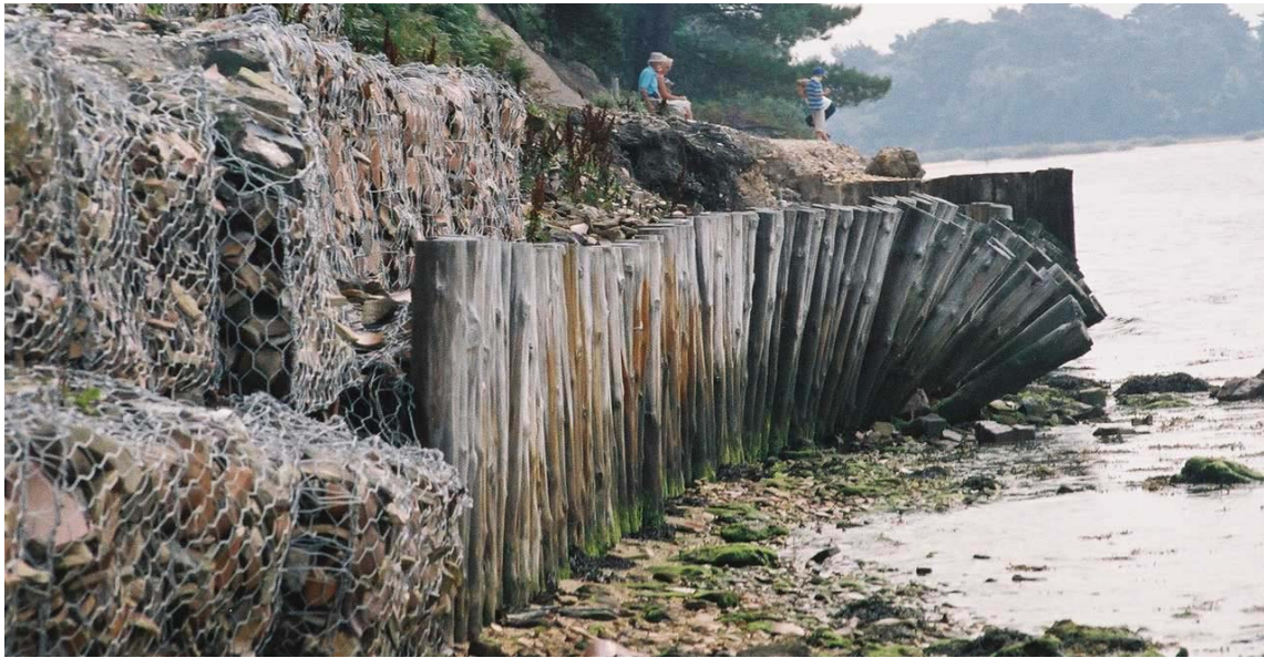
Figures 4.2.5 and 4.2.6: Ineffective, Ad Hoc, and Damaging Structural Sea Defences on Brownsea
