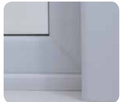
Welded Bottom Rail
