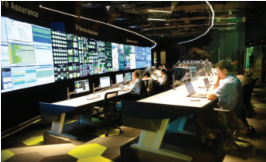
2017 saw Singapore pay-TV operator StarHub move its TV headend into its new Hubtricity facility. An IP backbone connects StarHub channels from integrated receiver decoders to the encoder farm, while bypassing the SDI baseband router. As the transition to IP continues to gain pace, expect more real-world deployments of both hybrid IP and full IP systems.
