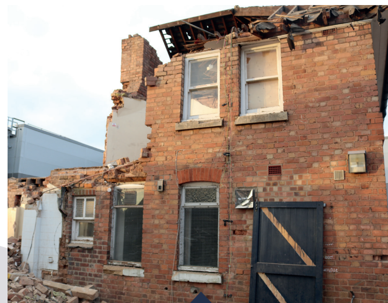
Demolishing the old building to make way for a new cadet centre in Hinckley.
