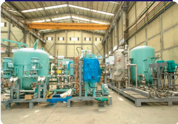
FRESH WATER SUPPLY PLANT
