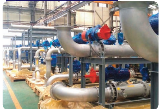
FRONT PIPE SKID
