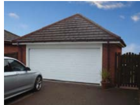
Roof carefully propped, old doors and brick pillar removed, new structural galvanised steel beam installed, 16'0" wide Hormann automatic sectional overhead door installed.
