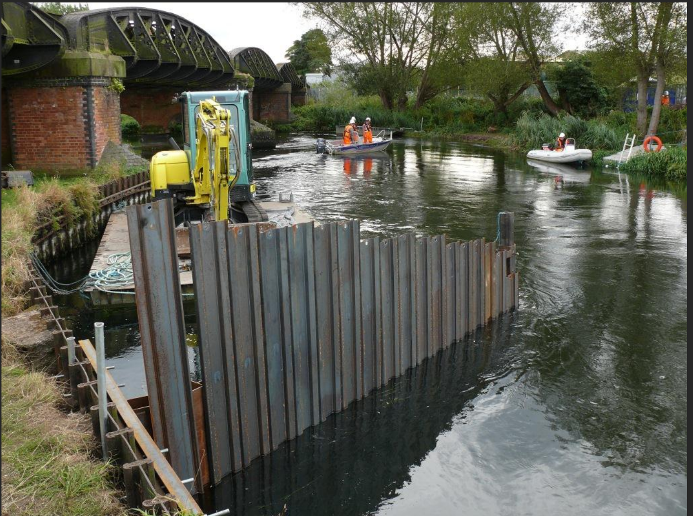
With the deflector plate installed, the silt curtain could be attached and work commence
