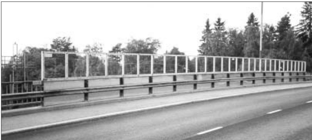
Electricity protection on railway bridge
