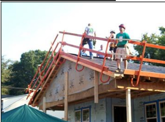
Temporary guardrails around roof.
