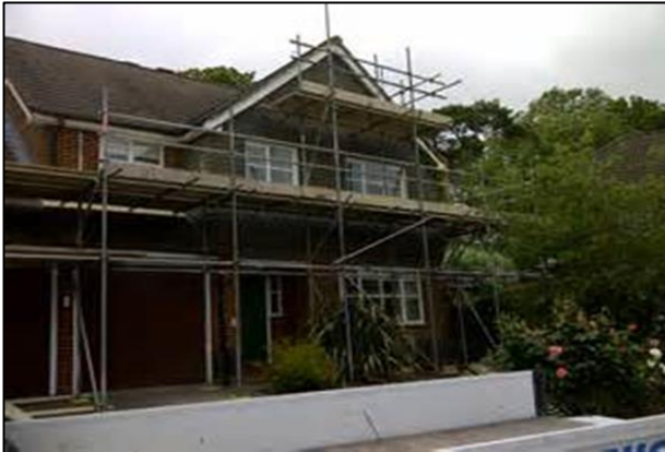
Traditional scaffolding with double guardrails and wooden toeboards to prevent person using from being able to fall.
