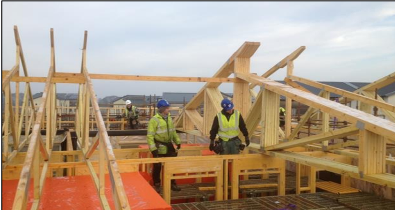
Elimination of fall risk by temporary false floor.
