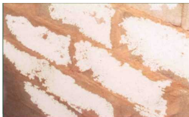
Figure 6.5 Remnants of asbestos on breeze blocks
