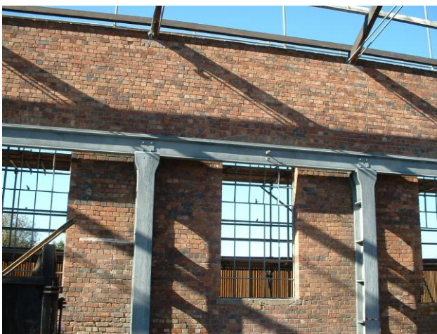
The cast-iron support columns before the roof was put on. These columns supported the original overhead crane.
