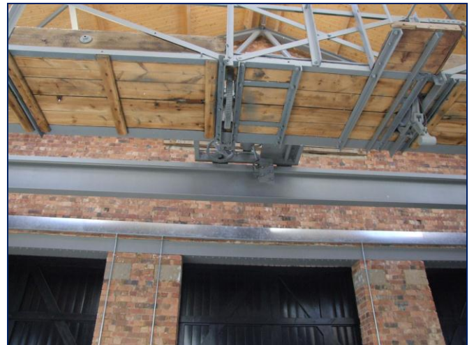
The original crawl-plank on the overhead crane were cleaned off and re-fitted onto the framework
