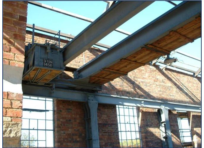
A view showing the crane resting on the H-beams supported by the vertical cast-iron columns.
