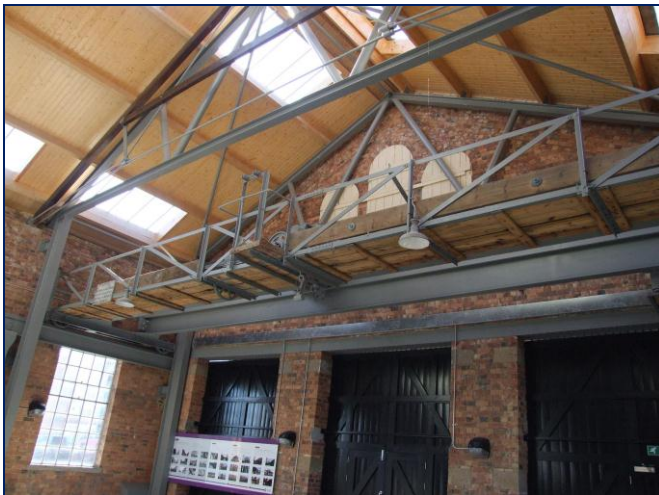
This view of the crane in May '09 shows the roof timbers and skylights now in place
