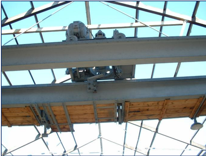
The crane was blast-cleaned and zinganned in '07 before the roof had its new timbers and glass skylights fitted.
