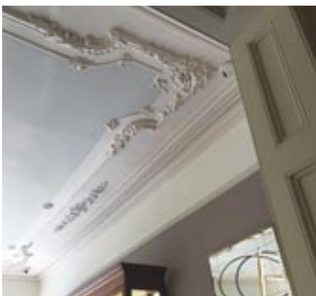
Original ceiling that was hidden in the Georgian House, now Optica Dublin
