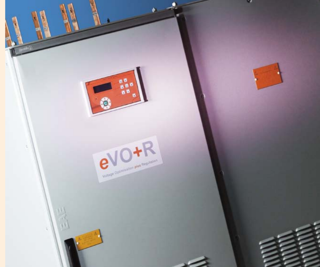
Left: Voltage management systems – such as voltage optimisation (VO) – deliver savings across the whole building rather than just individual electrical motors.
