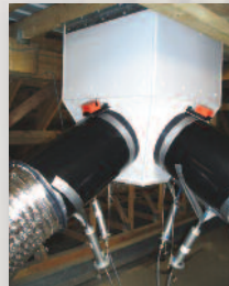
Sonic anemometers monitoring wind flow and direction within an Airscoop
