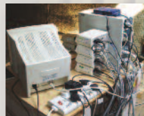
Data logger/collection of wind speed and flow and temperature
