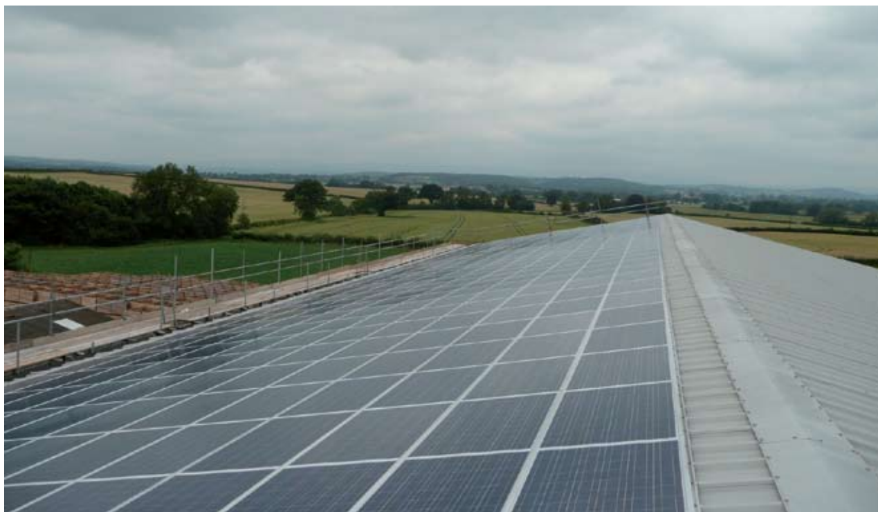
Dewsall Court SPV installation
