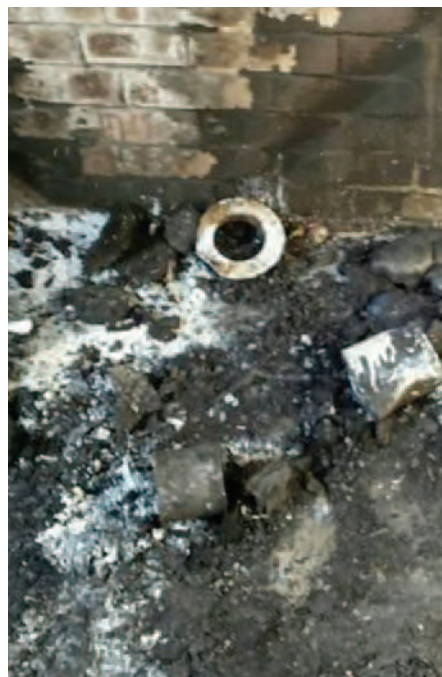
The aftermath of a fridge freezer fire.
