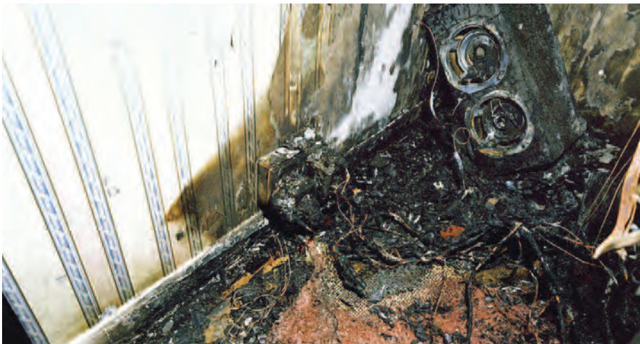
Overheated sockets: a clear example of the fire risk of an overloaded electrical circuit and its multiple plugs in a twin socket. On average, there are still approximately 25,000 UK fires of electrical origin each year.
