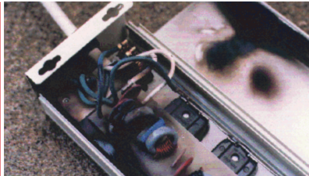
Burn marks inside a typical MOV suppressor.
