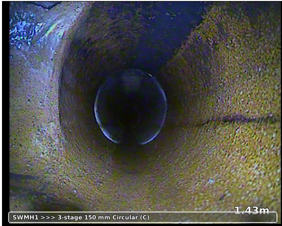
, 00:00:16, 1.43m Junction from/at 9 o'clock diameter: 150 mm
