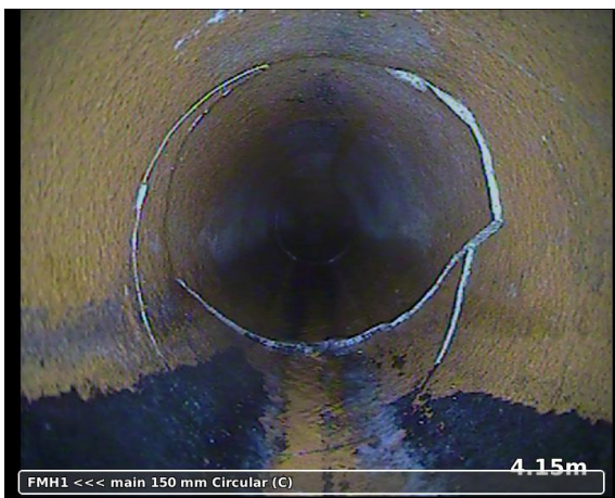
, 00:00:47, 4.15m Cracks multiple from/at 1 o'clock to 12 o'clock
