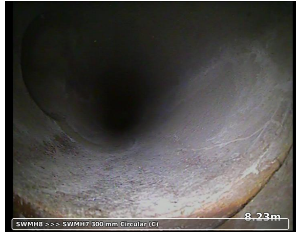
, 00:00:54, 8.24m Junction from/at 9 o'clock diameter: 150 mm
