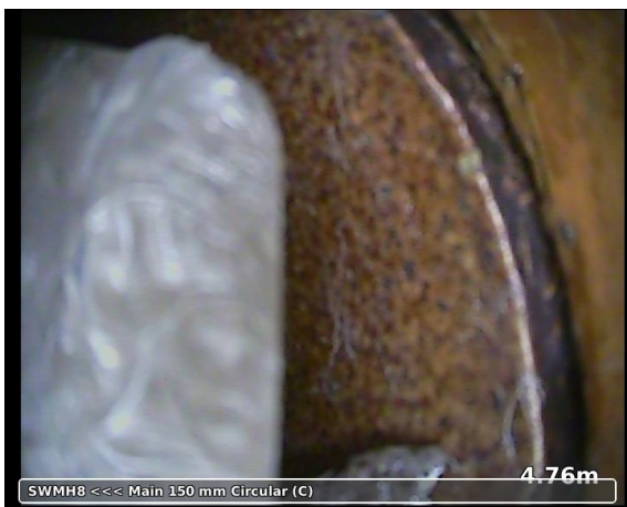
, 00:01:25, 4.76m Survey abandoned / Enters outlet of storm drain
