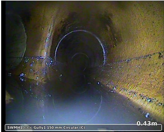
, 00:00:22, 0.43m Junction from/at 9 o'clock diameter: 150 mm
