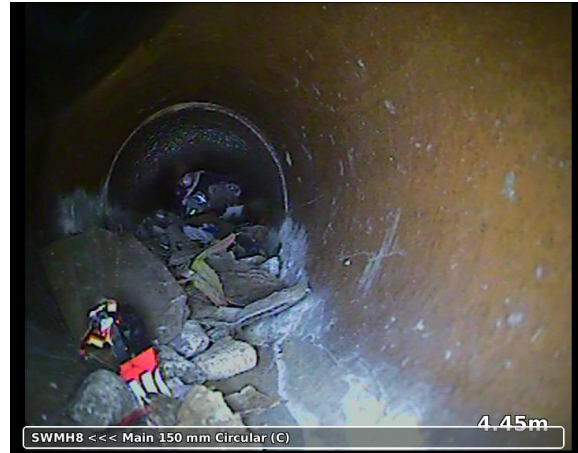
, 00:01:19, 4.45m Junction from/at 10 o'clock diameter: 150 mm
