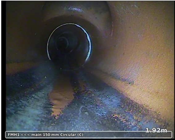
, 00:00:21, 1.92m Junction from/at 12 o'clock diameter: 150 mm
