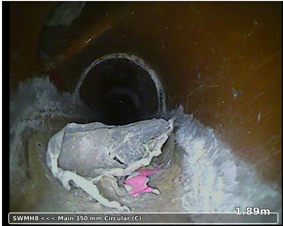
, 00:00:47, 1.89m Junction from/at 10 o'clock diameter: 150 mm
