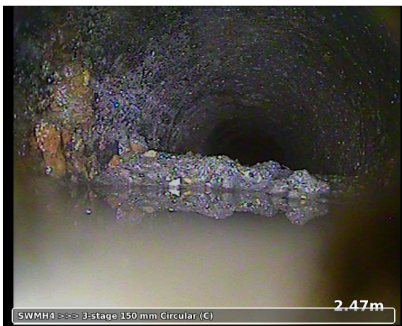
, 00:00:32, 2.47m Survey abandoned / Water level in interceptor too high
