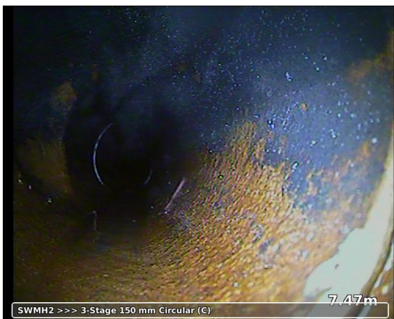
, 00:01:01, 7.47m Junction from/at 9 o'clock diameter: 150 mm / RWDP
