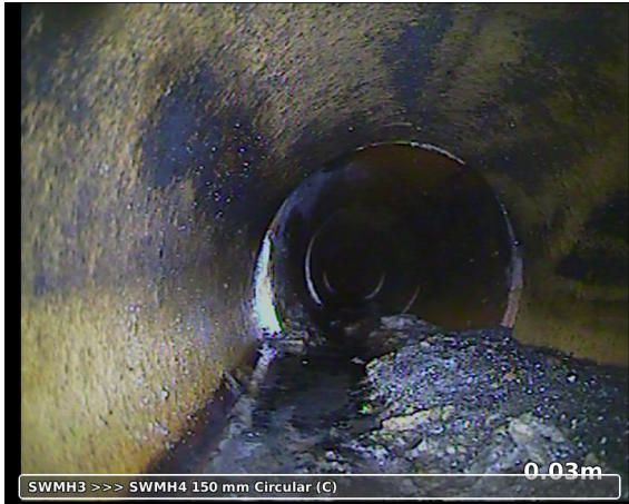
, 00:00:21, 0.03m Attached deposits other from/at 4 o'clock to 7 o'clock 20 % cross-sectional area loss
