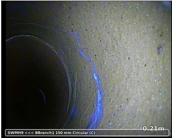
, 00:00:12, 0.21m Fracture circumferential at joint from/at 1 o'clock to 12 o'clock
