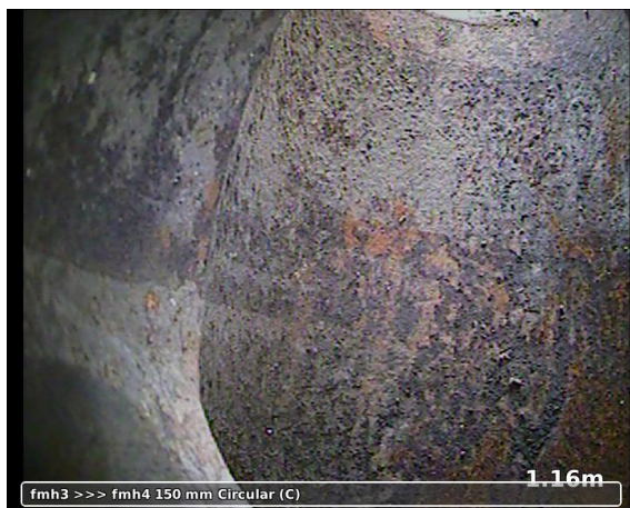
, 00:00:54, 1.16m Finish node type manhole reference number: fmh4
