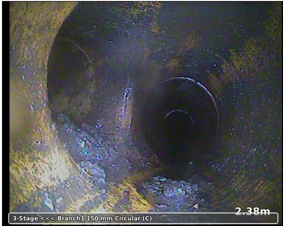
, 00:00:46, 2.38m Junction from/at 9 o'clock diameter: 150 mm
