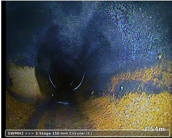
, 00:00:26, 3.54m Junction from/at 9 o'clock diameter: 150 mm / RWDP
