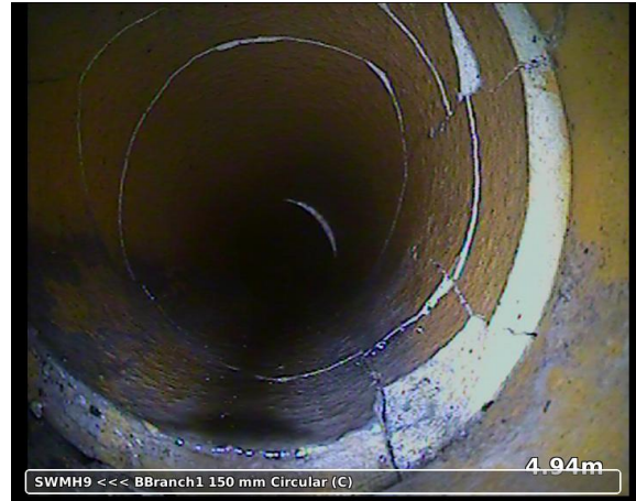
, 00:00:35, 4.94m Cracks multiple from/at 1 o'clock to 12 o'clock
