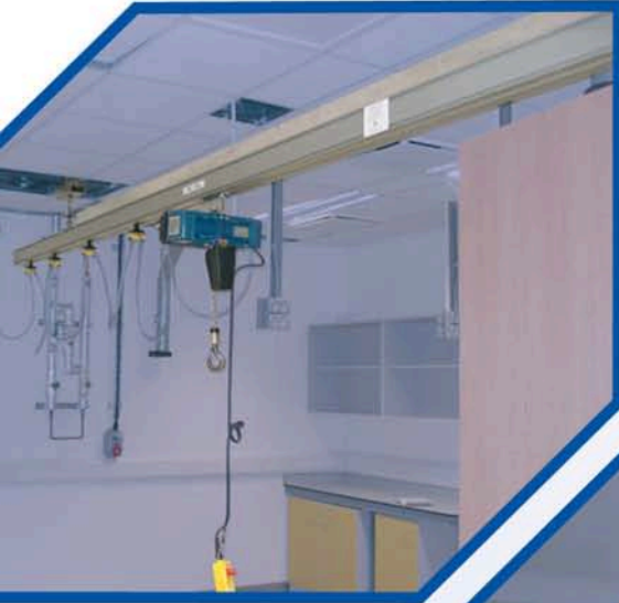
Ceiling mounted monorail with electric hoist.
