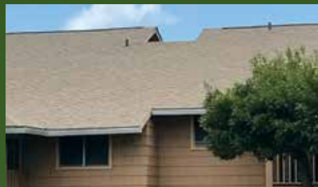
Waiau Garden Villas are topped with Malarkey’s Highlander NEX Golden Amber. PHOTO COURTESY MALARKEY ROOFING PRODUCTS
