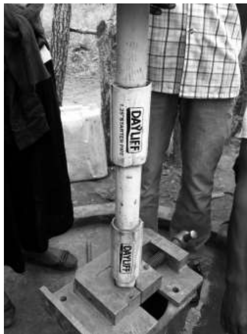
Figure 6. 1¼" PVC riser pipe fitted to an India MkII pump at Angodingod
