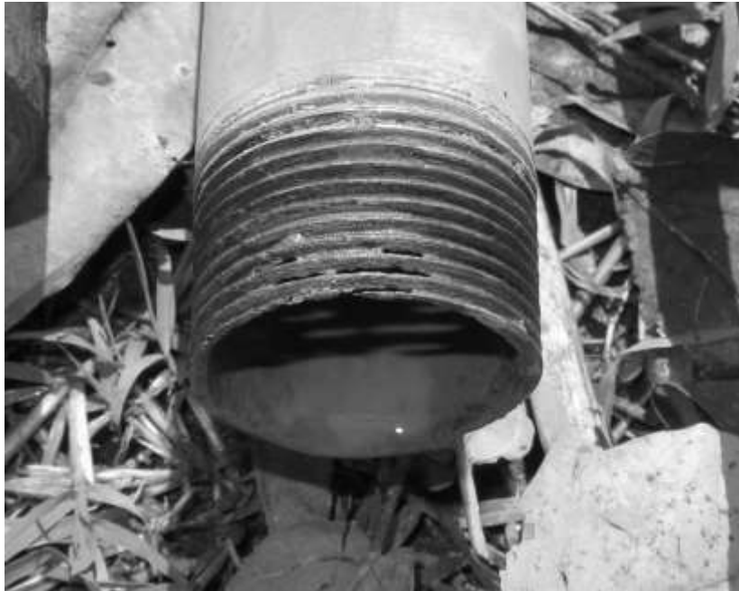
Figure 2 Threads on riser pipe at Odengelo, 1 year after installation
