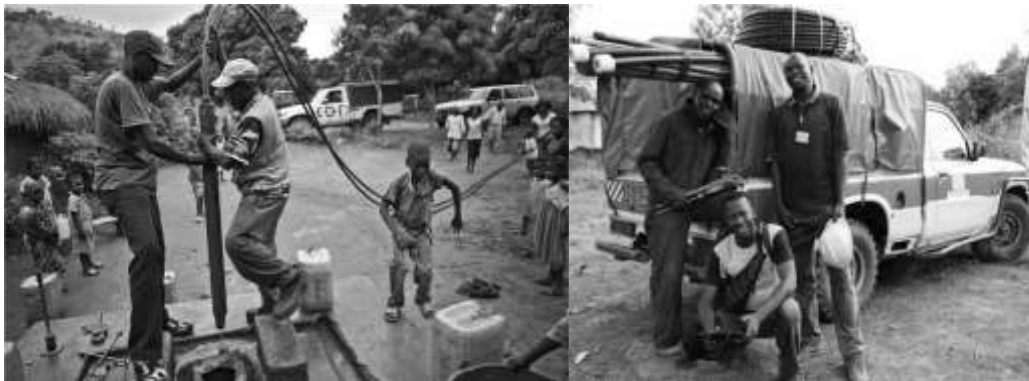
Figure 1. Above left, circuit-rider team pulling a pump out. Above right, circuit-rider team members with their truck, stocked with hand pump replacement parts.
