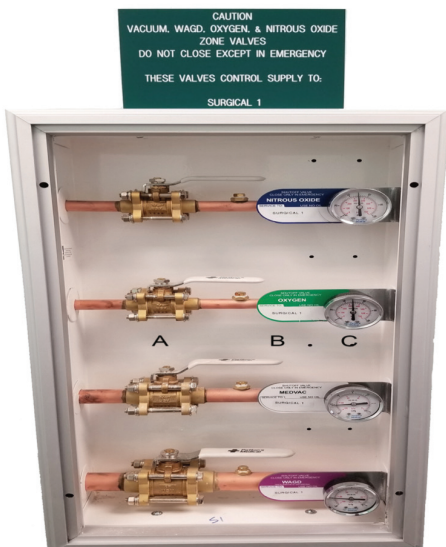
Figure 2: Zone Valve Box: A – 3 piece full port shut-off valve, B – Zone Valve Assembly label, C – Patient side vacuum/pressure indicator gauge.
