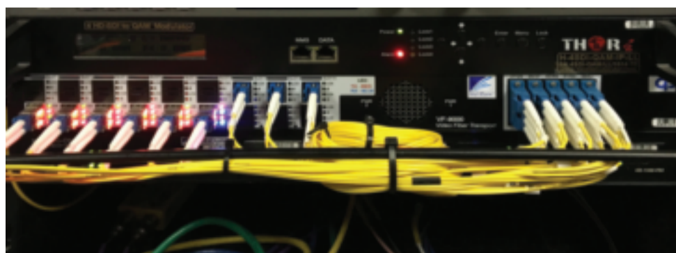
CP Communications, a US-based solutions provider for live event production, has installed MultiDyne's VF-9000 bulk fibre transport system in its HD-11 and HD-21 production trucks.
