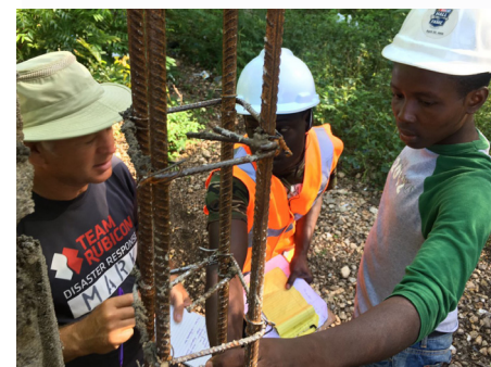
Team Rubicon UK works with local builders to put in place the structures for the new kitchens.
