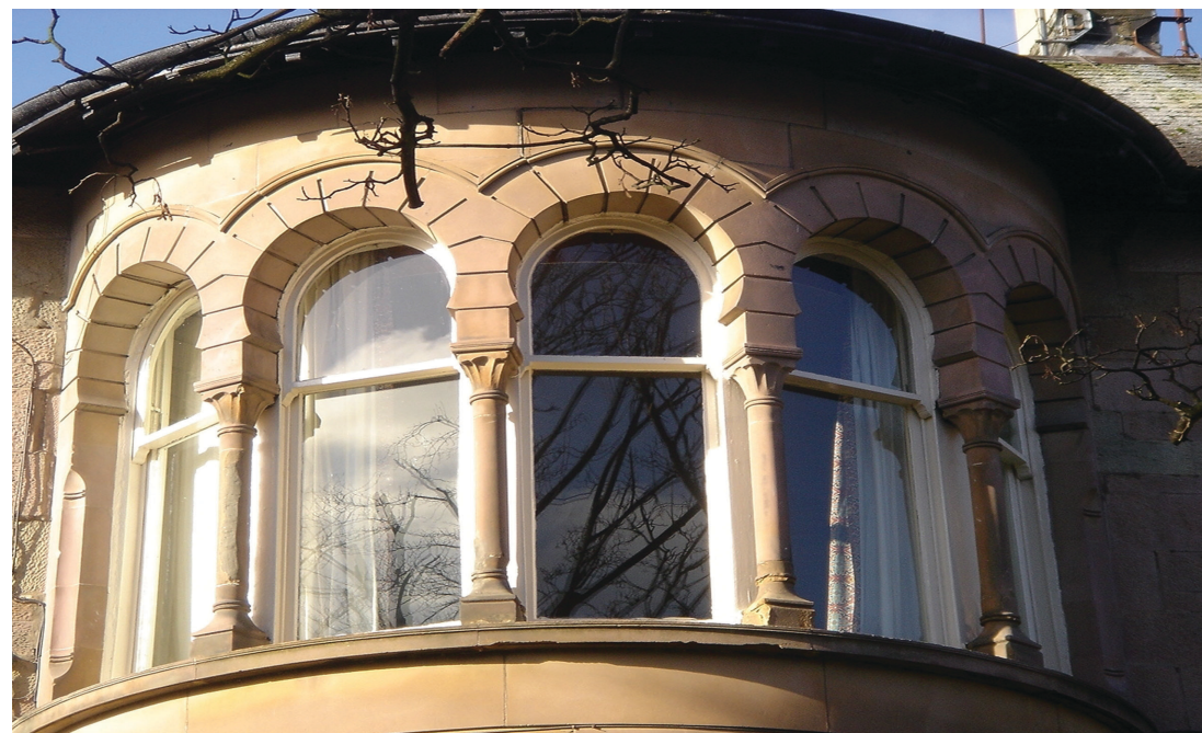
Top left and right: Historic windows before and after repair (courtesy of Glasgow City Heritage Trust) Bottom: West Pollokshields
