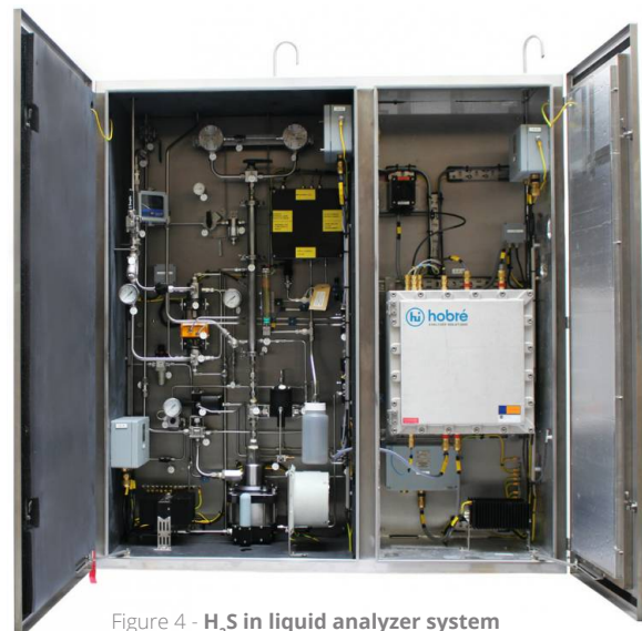
Figure 4 - H 2 S in liquid analyzer system
