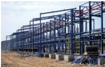
Railroad overpass for fuel oil discharge Marine commercial port Ust-Luga, Leningrad Oblast, Russia
