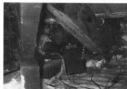
A moisture meter with a deep timber probe shows that despite the 'fresh' appearance of the fungal remains, the moisture content is below 8%. The dry rot is therefore very dead and the Rothound is proved right
